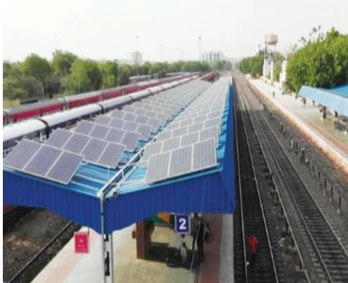
Figure 14: Solar panels install at a station roof top
