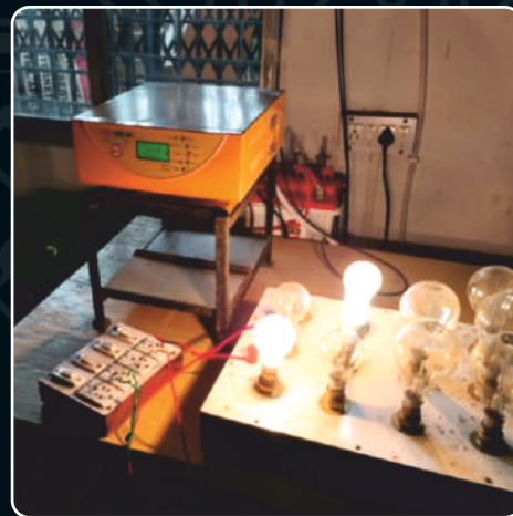
Battery ,Solar inverter and load
