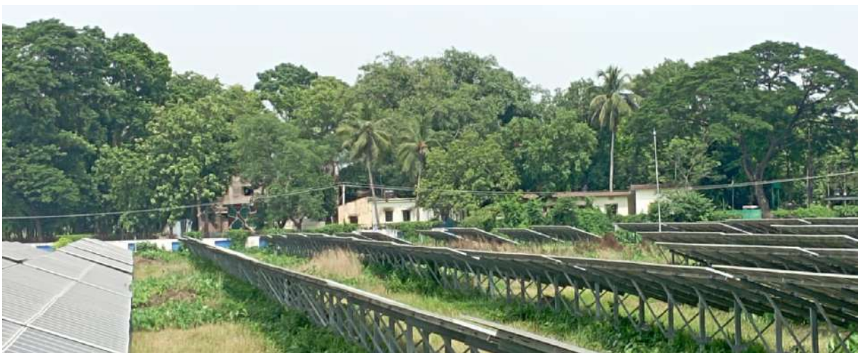
10MW Solar Project at Bhajanghat, Nadia
