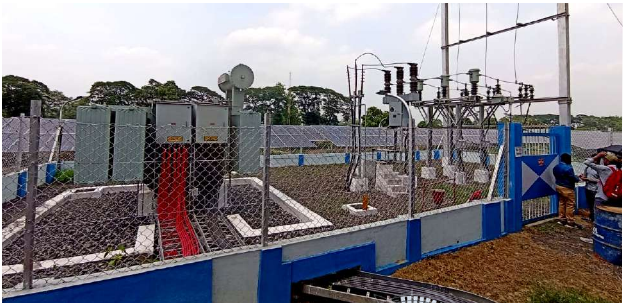
10MW Solar Project at Bhajanghat, Nadia
