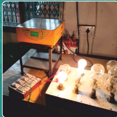
Battery ,Solar inverter and load
