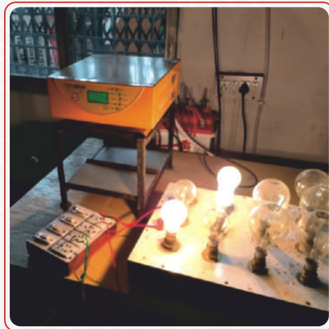
Battery ,Solar inverter and load
